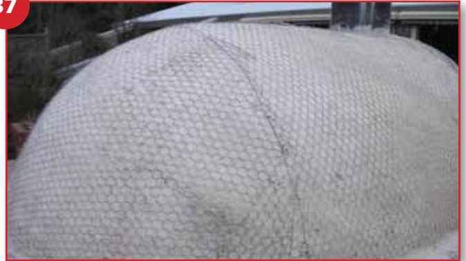
After allowing a drying period of 1 day, cover with chicken wire securing with staples supplied
