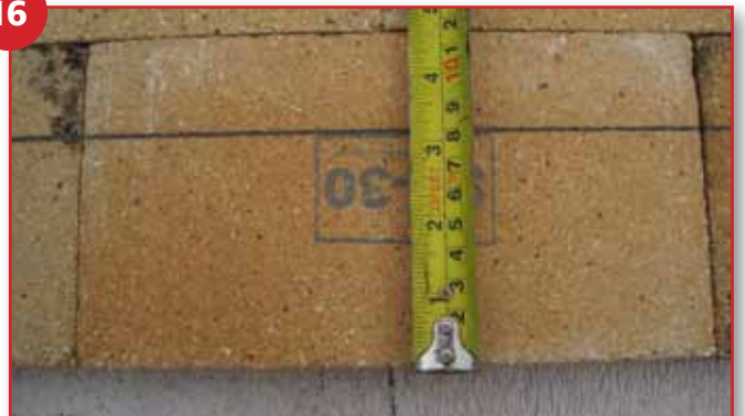
From the front row of fire bricks measure back 80mm and draw a line as pictured
