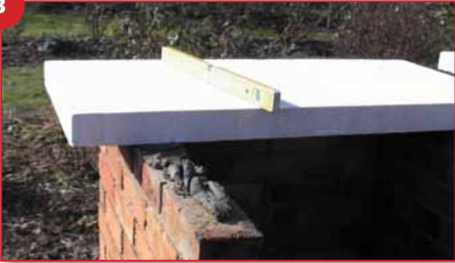
Place hebel on base allowing 100mm over hang to both sides and back
