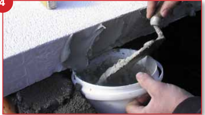
Mix up approximately 1/4 of the cement based glue to a thick paste and apply to hebel inner edge
