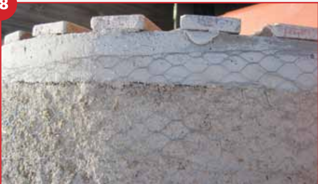
Bring chicken wire on to archway as pictured, and up to (not against) the flue
