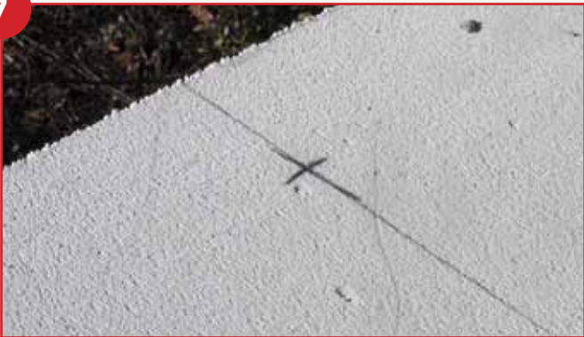
Mark a cross line on your centre line 120mm from the back edge of the hebel
