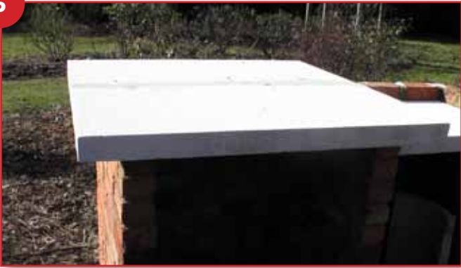
Bring the two hebel blocks together, smooth out any excess glue with trowel
